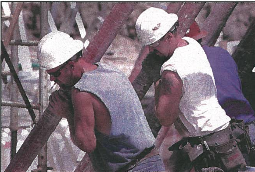
Thomas Conrad, left, of Waukegan and Jon Stephens, right, of Antioch hold support posts for a cement panel at the Fountain Square water tank project on the site of the former Fun Harbor.
